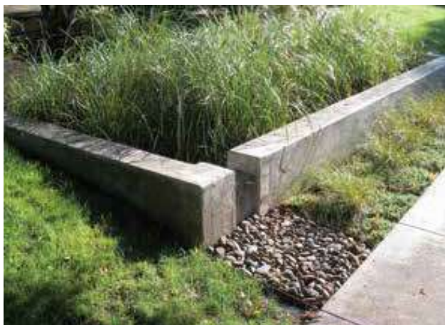
Fig16. Reference - outlet from Bioretention system
