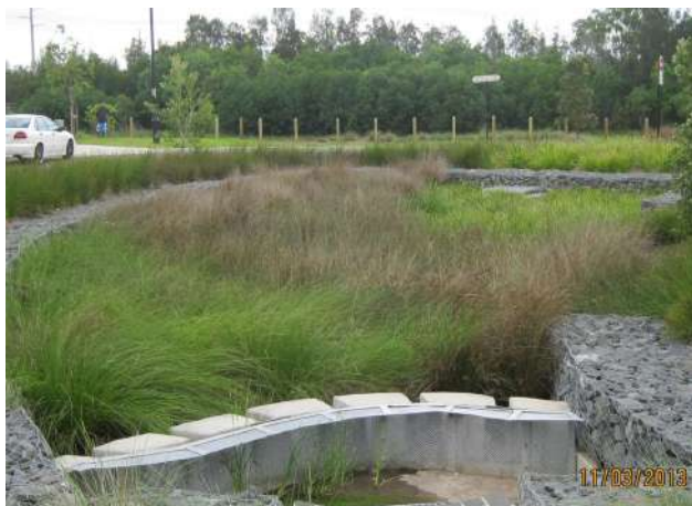
Fig 15. Reference - Inlet of Bioretention pond
