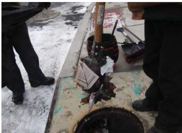
Fig 4.21. Reference - Cleaning of pretreatment device
