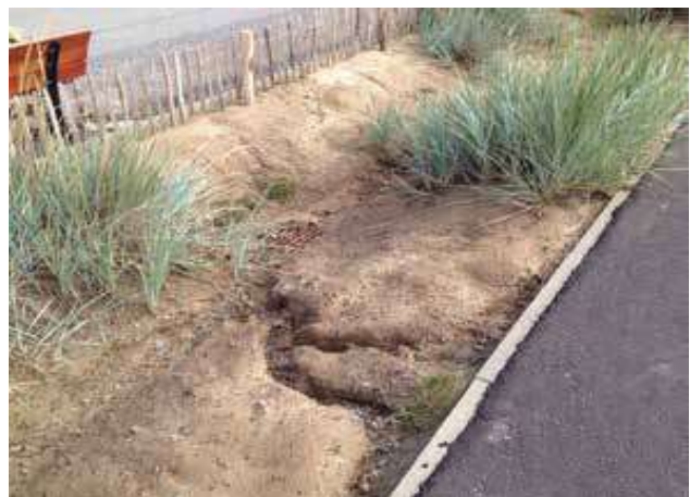
Fig 3.4. Reference - Absence of erosion protection before vegetation
