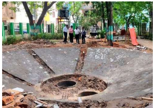
Fig. ii. Recharge pit in a constructed Sponge Park by Greater Chennai Municipal Corporation
